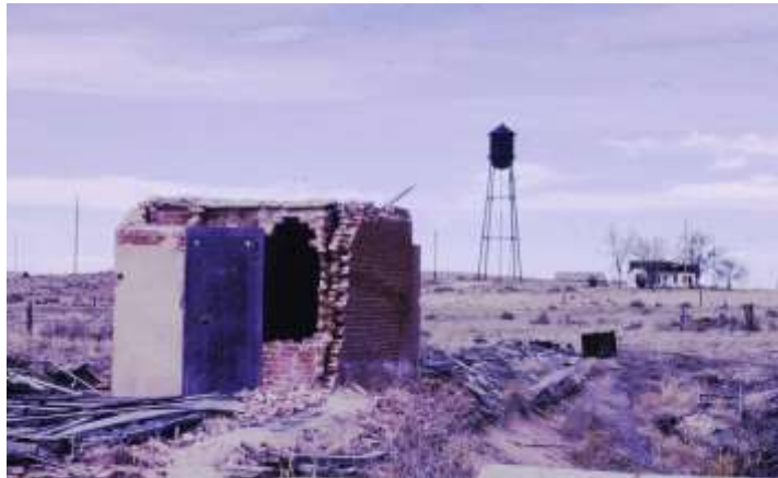
Remnants of a bank with the ever-present water tower in the background.
